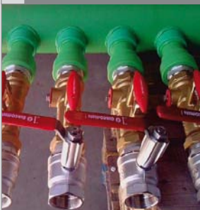
8 Distribution manifolds for geothermal application
