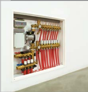
6 Distribution manifolds for radiant floor and wall
